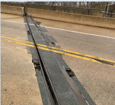
Damaged backwall/approach slab concrete and damaged expansion joint
